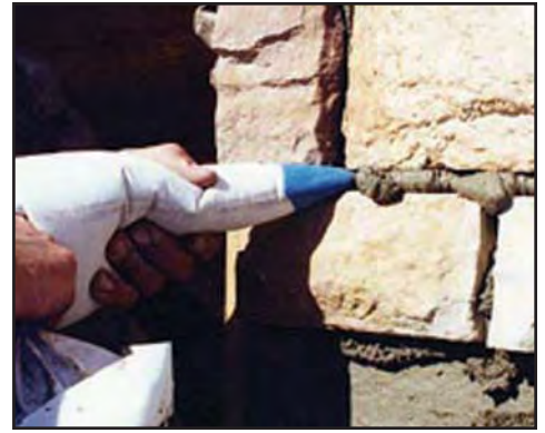
3. Fill the grout joints. Make a fist and push into the bag to force mortar into the joints.
