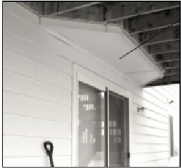
Exterior soffit appeared to be tightly fit
