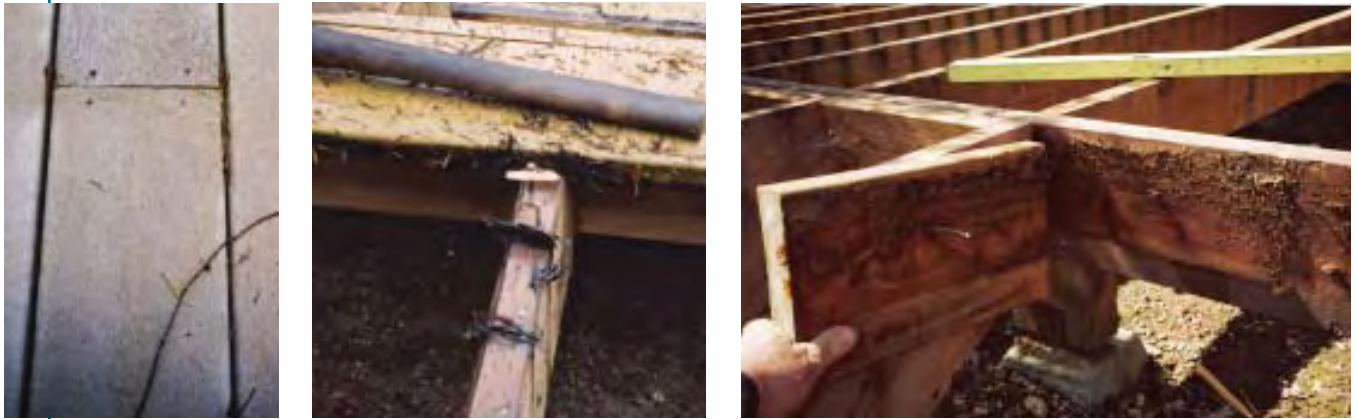
Figure 6. Most carpenters space deck boards too tightly (left), leaving enough room for debris to get in but no way to clean it out. On this deck, organic matter collected at every gap and joint (center), as well as between a rim joist and blocking that landed under a gap in the deck boards (right).
