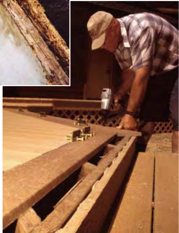
Figure 2. On this deck, water got between the fascia and rim, partially rotting the fascia and completely destroying the rim (above left). When the fascia was removed, the rim collapsed. Here (above), on a pressure-treated frame, the author installs composite decking that will completely cover the fascia and rim, avoiding this potential collection zone. The lattice separating the fascia and rim joist will also help to drain away water.
