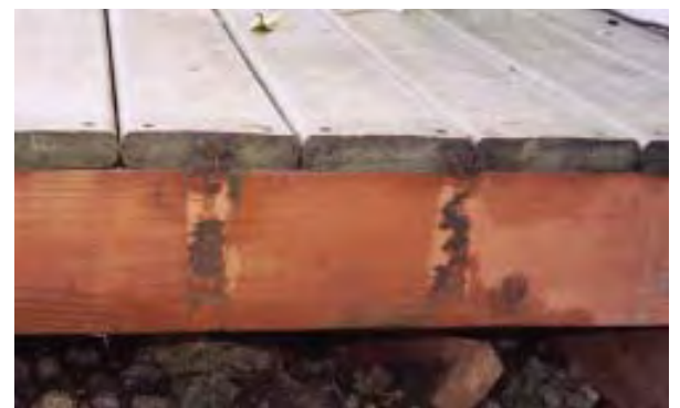
Figure 7. Nailing balusters to the rim joist creates pockets that trap moisture and debris, which can cause rot.
