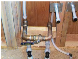
House water shut off under cabinet..
