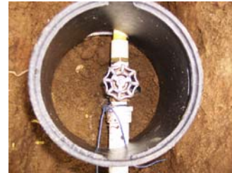
Water shut off valve in valve box, outside in ground.
