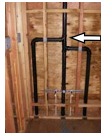
Vent connection of downstairs fixtures must be 6" above the overflow rims of fixtures on this floor.
