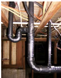
Bath tub drain with vertical vent.
