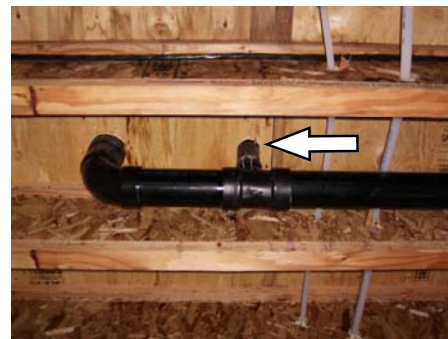
Vertical vent to wall above. Looking up at second floor, floor joist.
