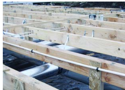
Under floor pipe up in joist space where it will be insulated
