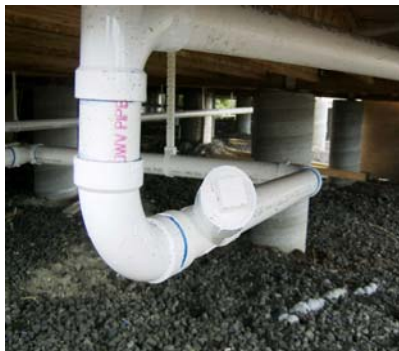
End of line cleanout. Cleanouts are required for change of direction over 135 degrees in horizontal turns. That's 1-90 degree turn and 1-45 degree turn.
