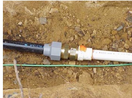
Connection of CPVC to Polybutylene. Polybutylene is to be used outside only. The black pipe.
