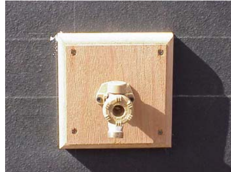
Outside frost proof hose bib with vacuum breaker.
