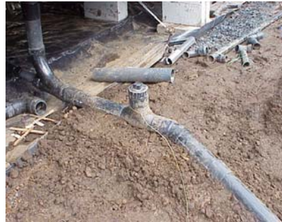
Two way cleanout outside of house is preferable or a end of line cleanout may be used. A sewer line must have cleanouts every 100 foot. Green tracer wire 18 ga. on sewer.
