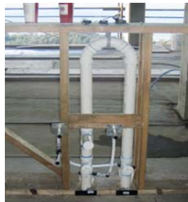
Loop vent to top of cabinet
