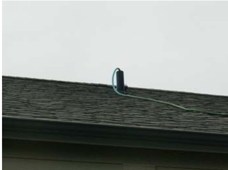
Hose in roof vent filling waste with water for test. Ten foot head of water.
