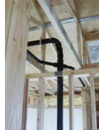
Vents connecting together in attic.
