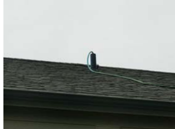
Vent 6" above roof. Never terminate vents in attic space. Hose for water test of the new waste system.
