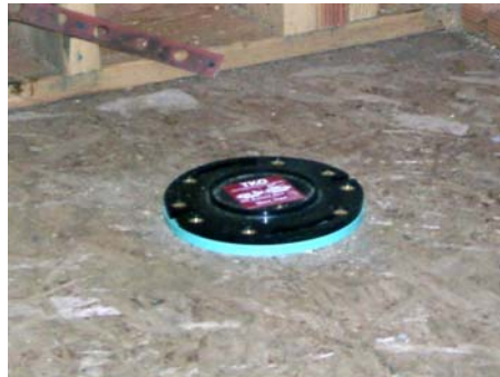
Toilet flange with brass screws holding it to floor. Cap for test. Blue spacer ring for sub sheeting.
