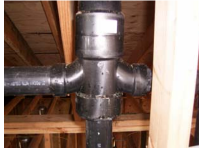
Double san tee. Used to connect two horizontal vents to a vertical stack. Fitting upside down.
