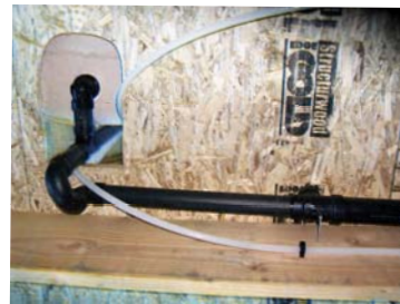
Bath tub drain with flat vent. Looking up at second floor, floor joist.
