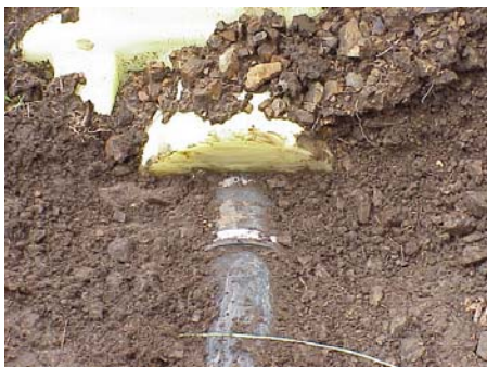
Connection of ABS waste pipe to septic tank using a Fernco rubber coupling.
