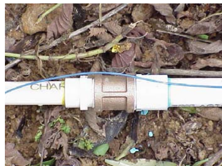
Connection of PVC to CPVC outside of house. PVC is not allowed to be inside of house.
