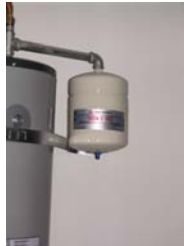
Expansion tank on water heater. This is used when there is a check valve on water service.
