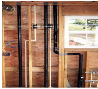
Mid-story strap waste, vents and water lines.
