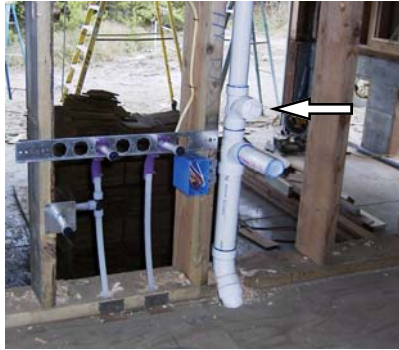
Cleanouts are required for the kitchen sink. Cleanouts on the second floor of the building are not required.
