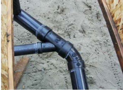
Y-fitting receiving waste from sink.
