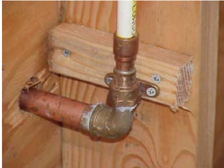
Flow Guard gold CPVC water pipe fastened to structure for hose bib outside.
