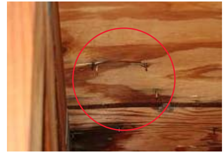
Figure 7 - Corroded roofing nails
