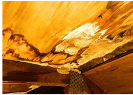
Figure 6 - Staining & damaged roof sheathing caused by water leaks
