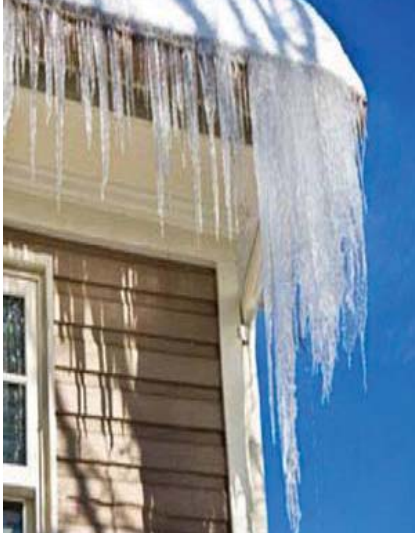
Figure 10 - Icicles on gutters may indicate ice dams
