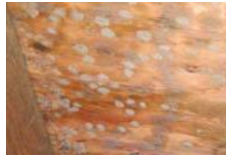
Figure 8 - Mold growing on the underside of the roof deck & supporting roof structures
