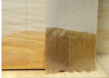
Figure 4 - Water being absorbed by paper towel & plywood sheathing
