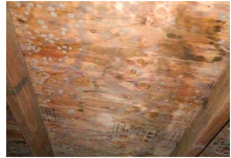
Figure 5 - Condensation on the underside of a roof deck
