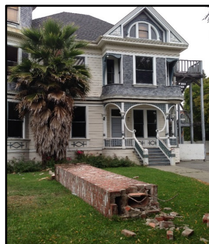
Figure 2: Chimney damaged in the South Napa Earthquake. Photo Credit: Janiele Maffei, CEA
