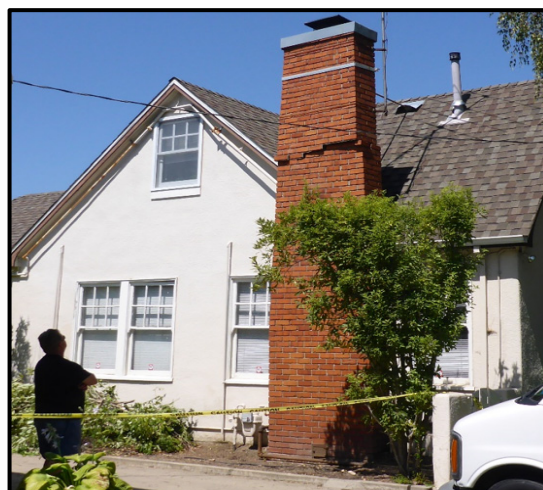
Figure 1: Chimney damaged in the South Napa Earthquake. Photo Credit: Exponent.
