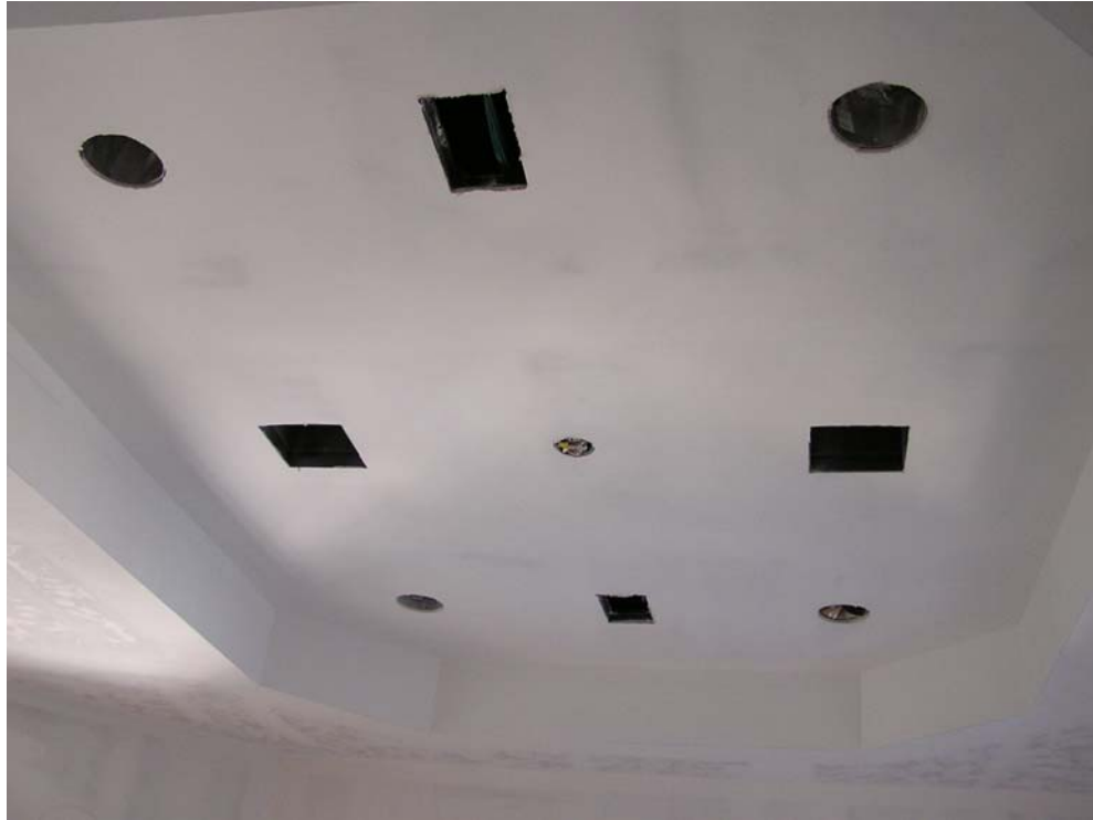
Photograph 1: Ceiling Penetrations – “Swiss Cheese Services”
