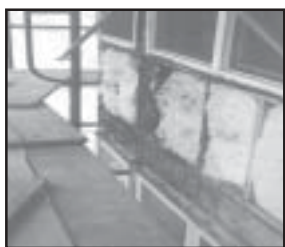
Failure of sheathing attachment to Substrate
