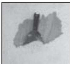
Finish not bonded to Base Coat
