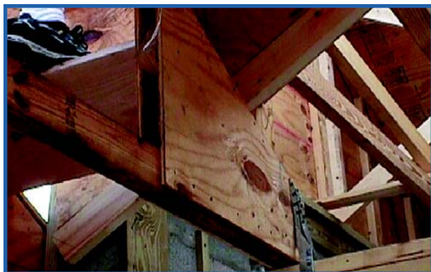
An example of a properly repaired truss after it was shortened four inches.
